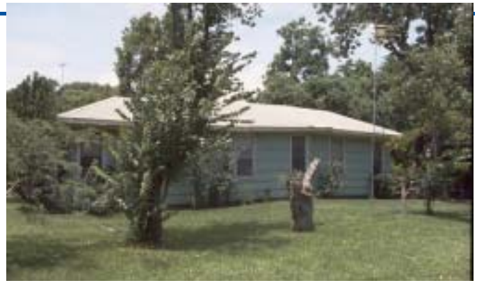
Residence impacted by subsidence. HGCSO photo
